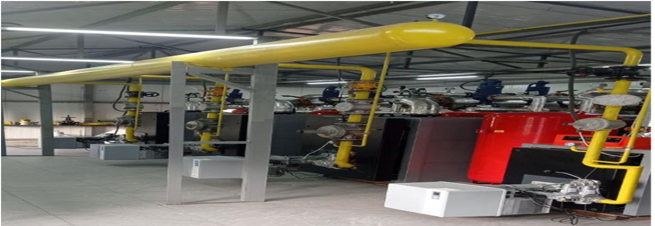
3. Heating system (UzSWLU)
