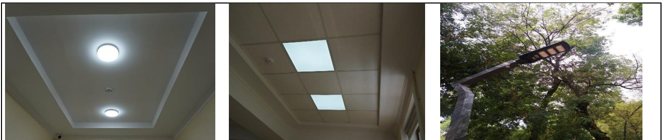
Example of Energy Efficient Appliances Usage: Use of LED lighting and lamps with light detection (UzSWLU)
