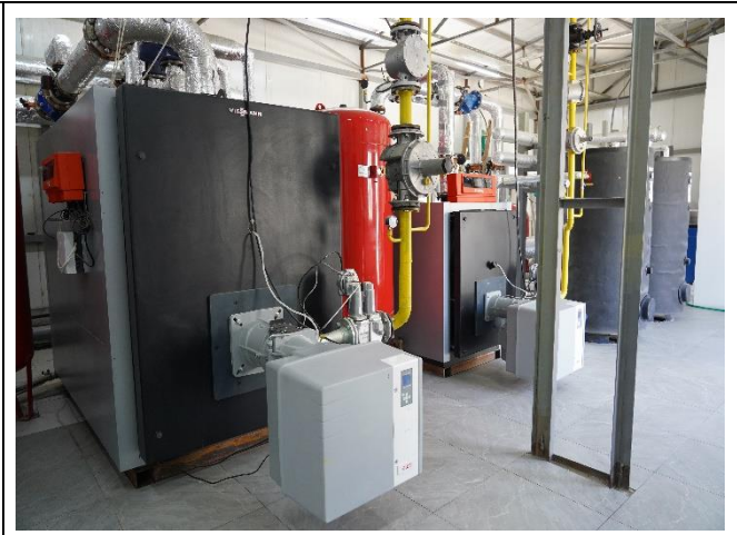
Heating gas boilers (UzSWLU)
