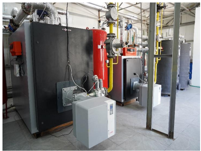
Heating gas boilers (UzSWLU)
