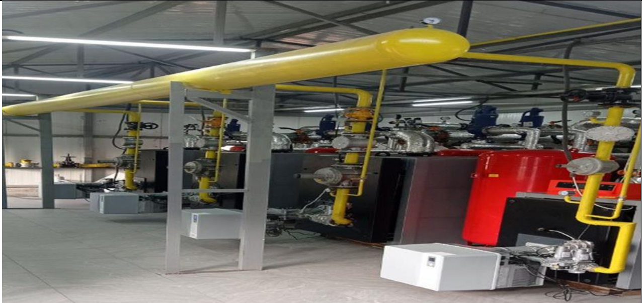
Water distribution equipment of the University (UzSWLU)
