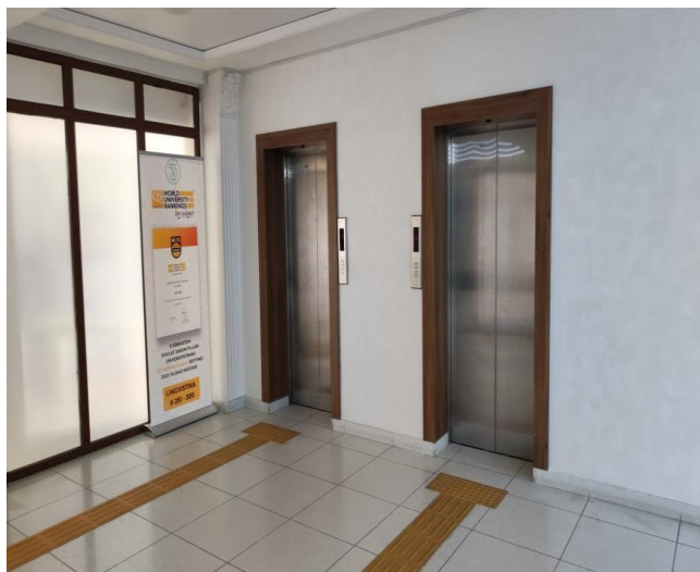
Elevator for students
