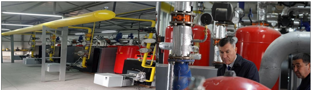
Water distribution equipment of the University (UzSWLU)
