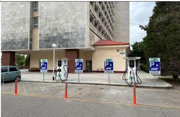
Electric-vehicle charging infrastructure
