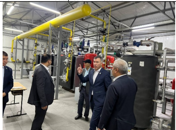
High-efficiency heating system
